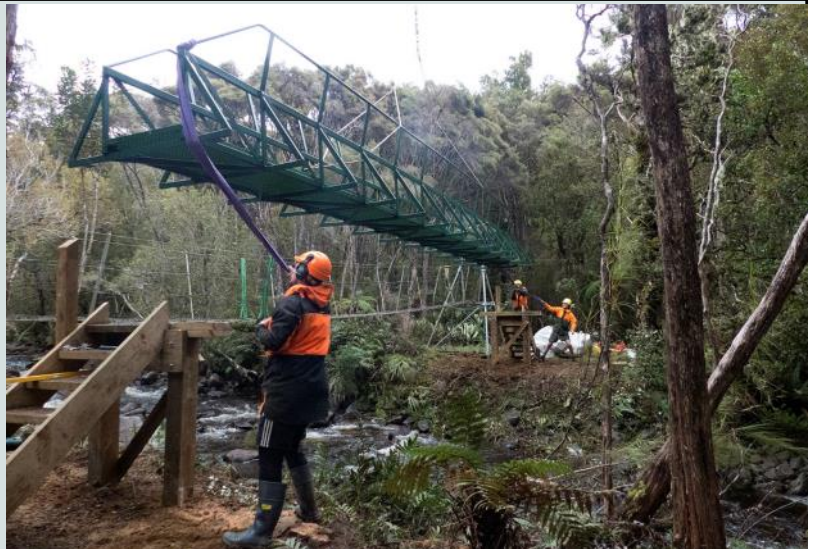
The new bridge at Christmas Village being lowered into place by helicopter
