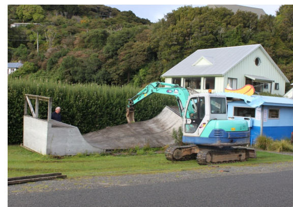
Bye-bye to the skate ramp! The removal is making way for the new community bowling green. Photo from Alina Atkins.
