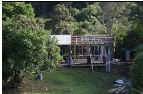
Work is currently underway upgrading and extending Port William Hut. The hut will remain closed to the public until the work is completed, which expected to be around the end of May.
