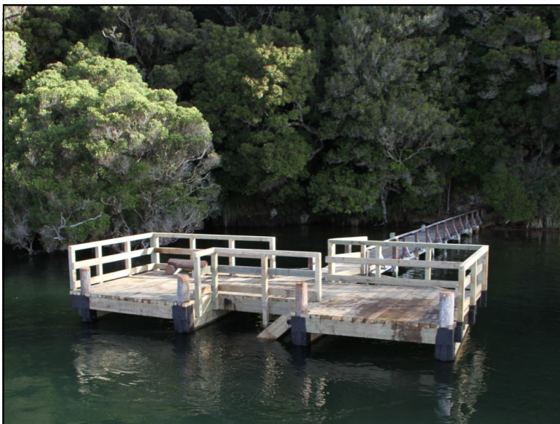
The new Fred's Wharf. Hats off to the hard-working pile-driving bollard swinging timber technicians behind this beautiful creation. Thank you Grim Davis, Greg Northe and Stu Ross.
